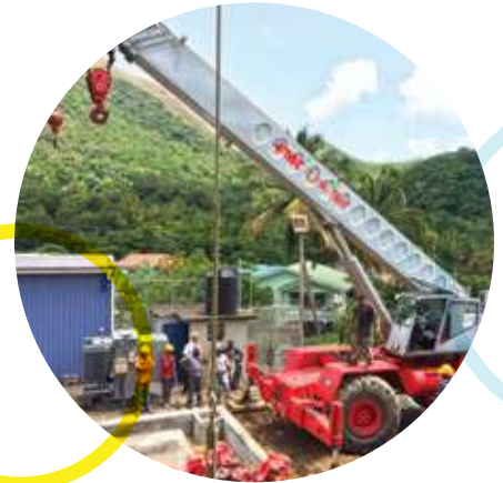
The Soufriere substation was re-commissioned following its shut down in May 2012. Work at the site involved replacing the damaged transformer and upgrading the protection system at the facility
